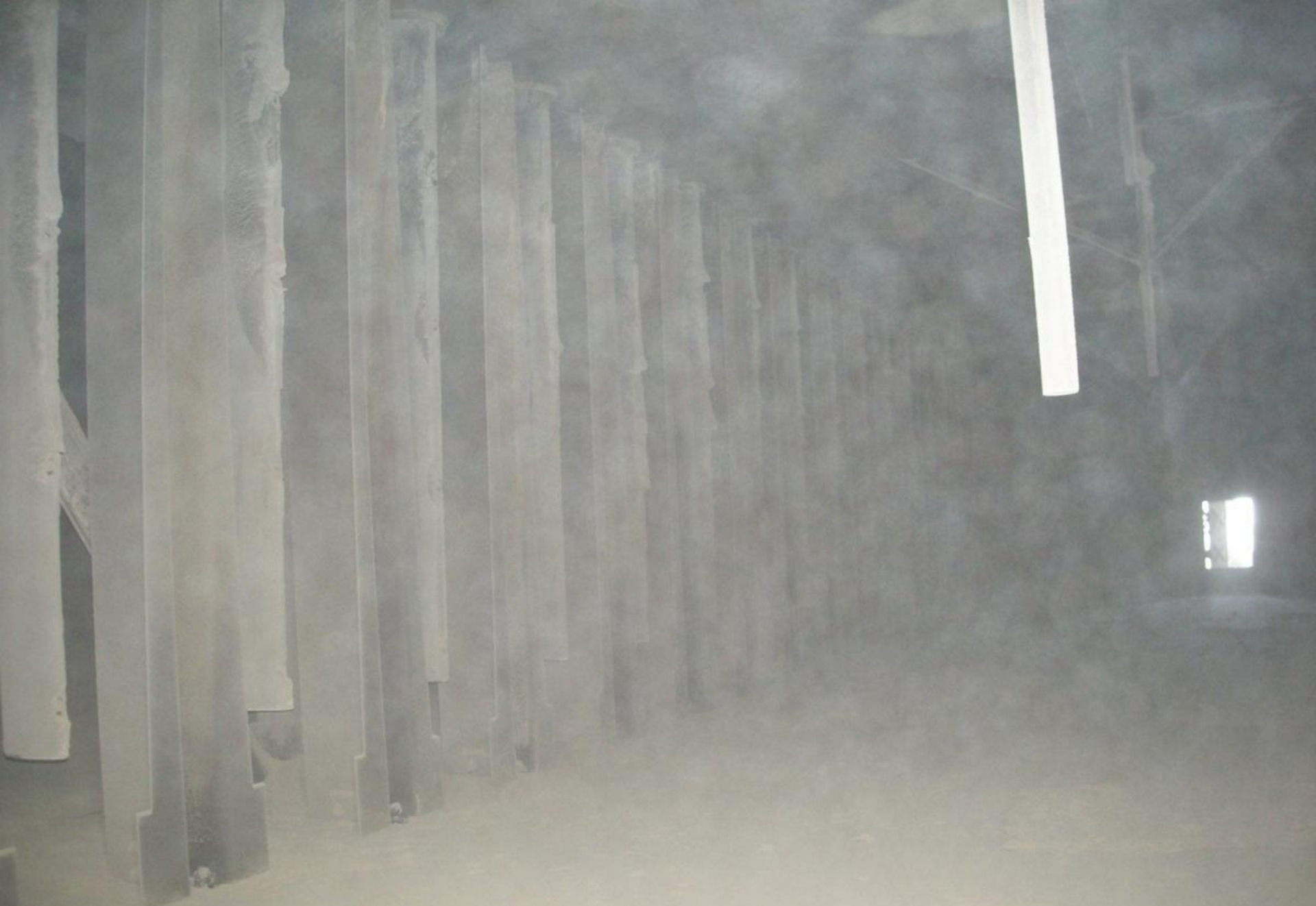
Injection Duct (Harding Street) – After 8 Months of Operation
